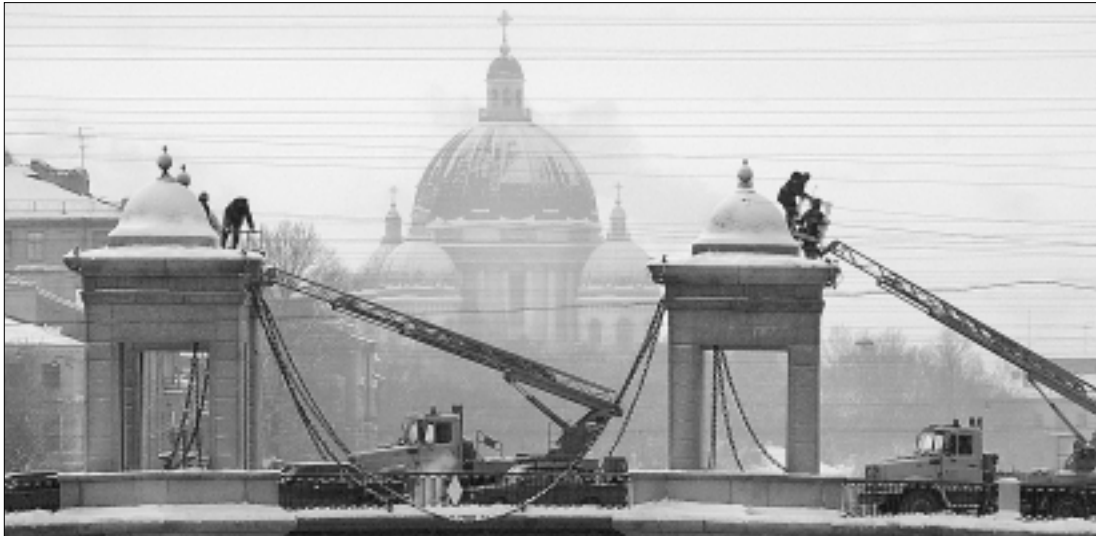
WORKERS REPAIR towers on St. Petersburg's Lomonosov Bridge in preparation for its 300th Jubilee celebrations this year. The Jubilee is drawing more foreign corporate interest in local businesses, says Dun&Bradstreet Nord Director Ila Vinnik.
